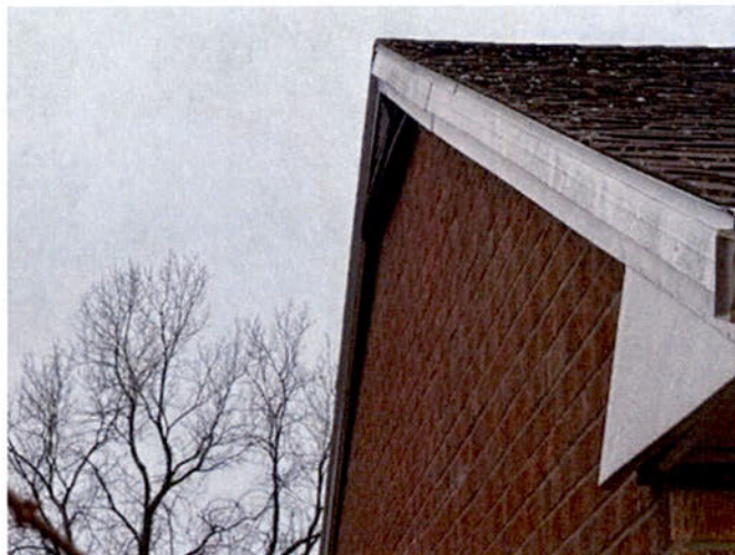
Close up look at the deflection.
