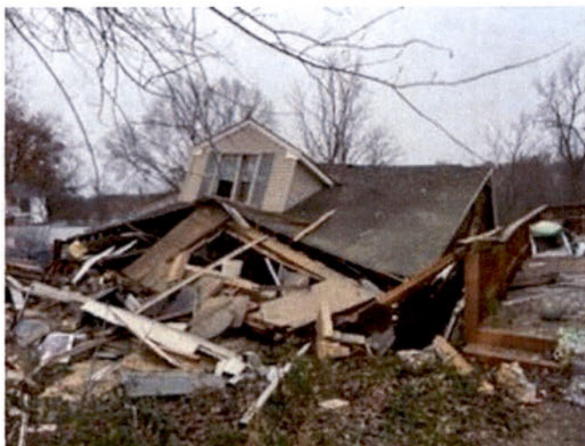
Alpha delta corner. The gas service was leaking somewhere in the ground near this area.
