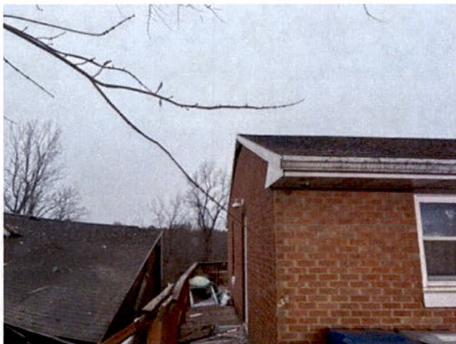
Possible deflection of the Delta side neighbor residence due to blast. Top of the gable end of the brick wall.
