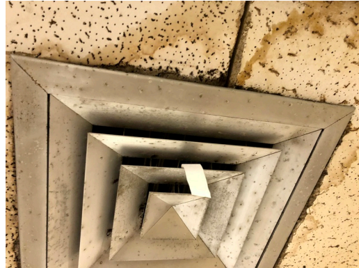
14. Stained Ceiling Panel and Diffuser
