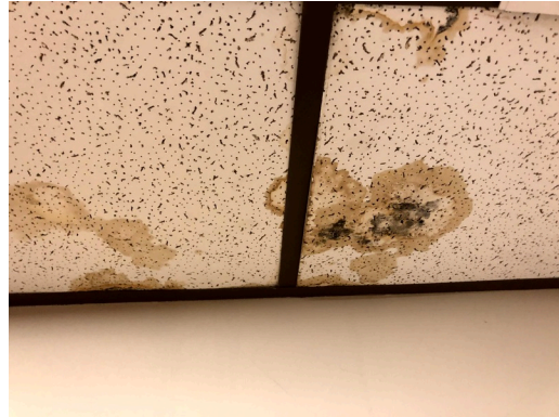
16. Stained Ceiling Panel (Locker Room)
