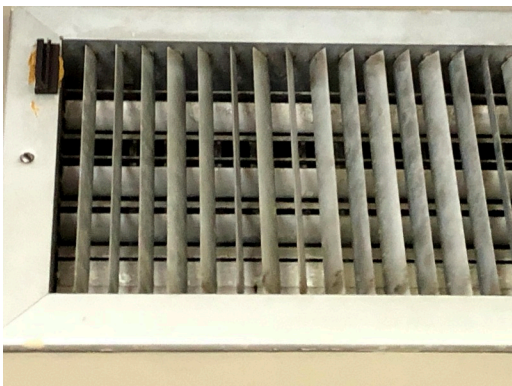
35. HVAC Supply Louver
