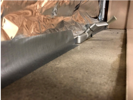
31. Dirt accumulation on Window Ledge
