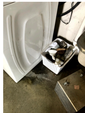
48. Water Accumulation and Staining in Apparatus Bay
