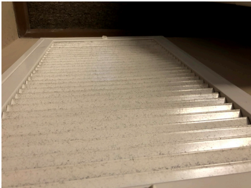
33. Dirt accumulation on HVAC Louver
