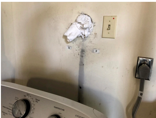
47. Former Dryer Vent Exhaust
