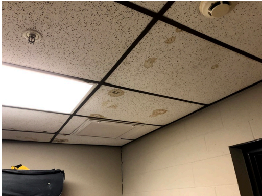
15. Stained Ceiling Panels (Locker Room)
