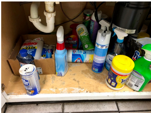
19. Previous Moisture Damage (beneath Kitchen sink)
