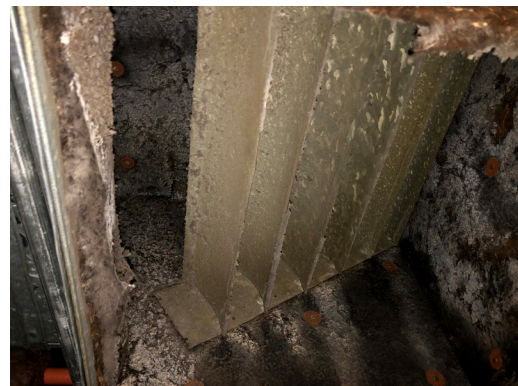
36. Interior duct insulation and dirt accumulation
