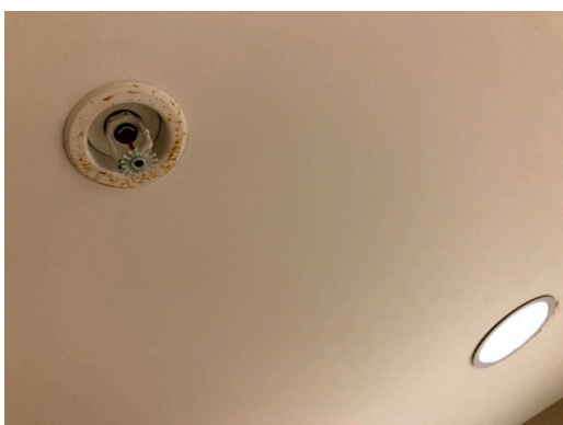
23. Fire Sprinkler rust in Shower area
