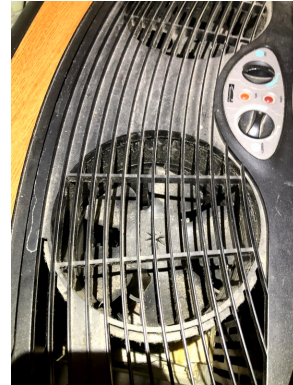
32. Dirt accumulation on Humidifier (Dormitory)
