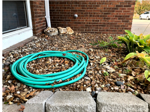
50. Poor drainage and landscaping
