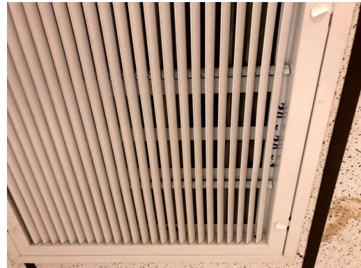
34. HVAC Return Louver and Filter
