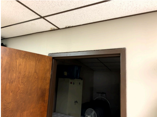
13. Stained Ceiling Panels (Kitchen)
