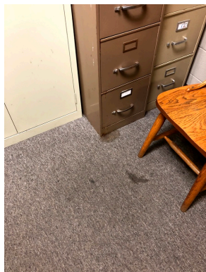
17. Stained File Cabinet and Carpet (Locker Room)
