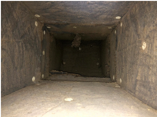
9. Kitchen/Dining - Interior Ductwork
