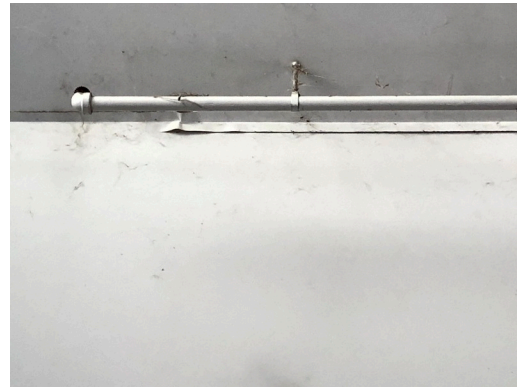
22. Apparatus Bay - ceiling drywall tape damage
