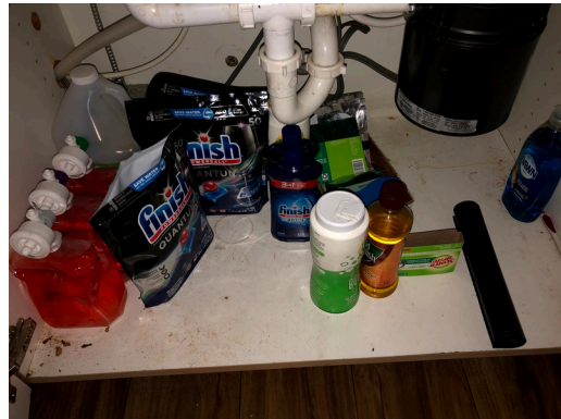
10. Kitchen - beneath sink
