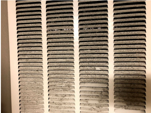
7. Kitchen/Dining - HVAC return louver
