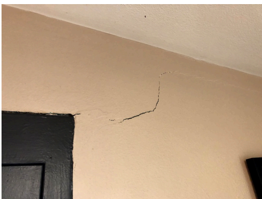
5. Damaged Wall (Living Room)
