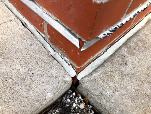
43. Exterior - weathered sealants
