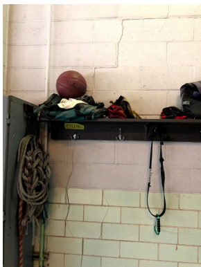
23. Apparatus Bay - damaged wall
