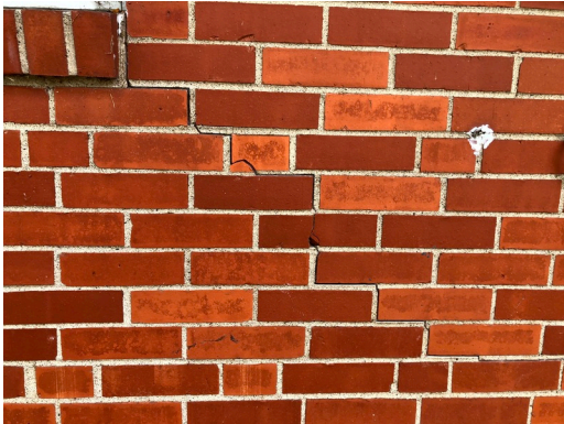
39. Exterior - Brick Damage
