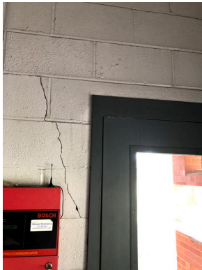
21. Apparatus Bay - damaged wall
