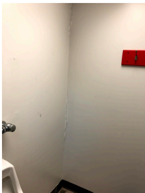
29. Bathroom - drywall tape damage
