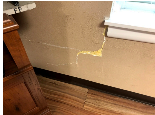
4. Damaged Wall (Living Room)
