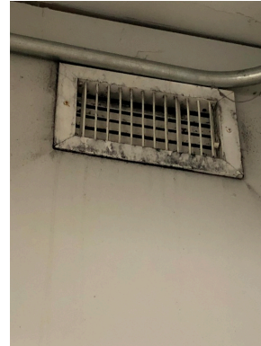
26. Laundry Room - HVAC louver
