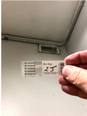
37. Laundry Room HVAC Louver - Location of Surface Sample 2J
