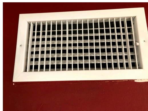
6. HVAC Louver (Living Room)
