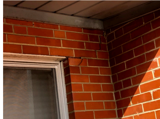
40. Exterior - Brick Damage
