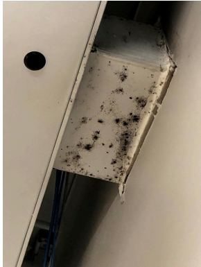
25. HVAC duct at doorway to laundry room
